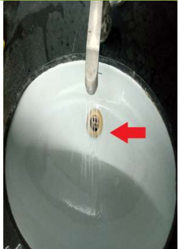
Tap water system with Reducer
